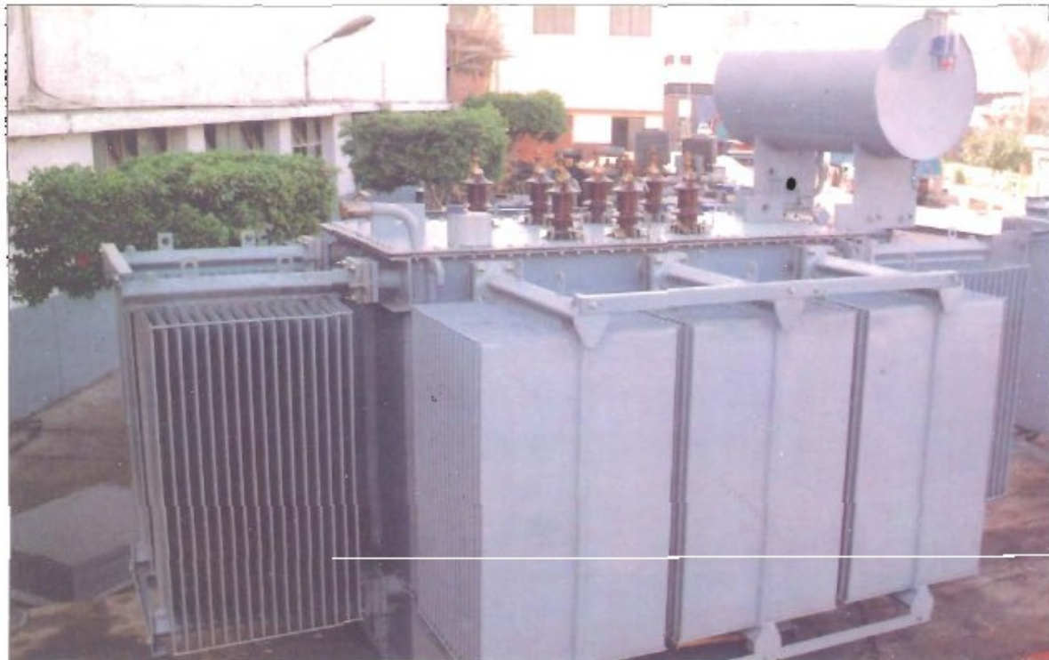
Transformer With Radiators Tank
